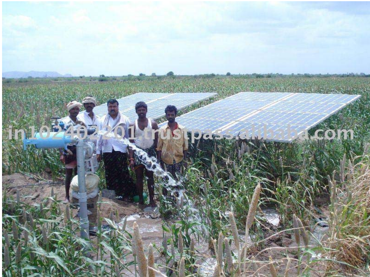
Power for Island agricultural irrigation system
